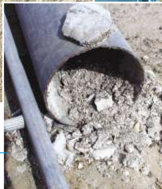
Deposits of CaSO 4 in a sludge pipe
